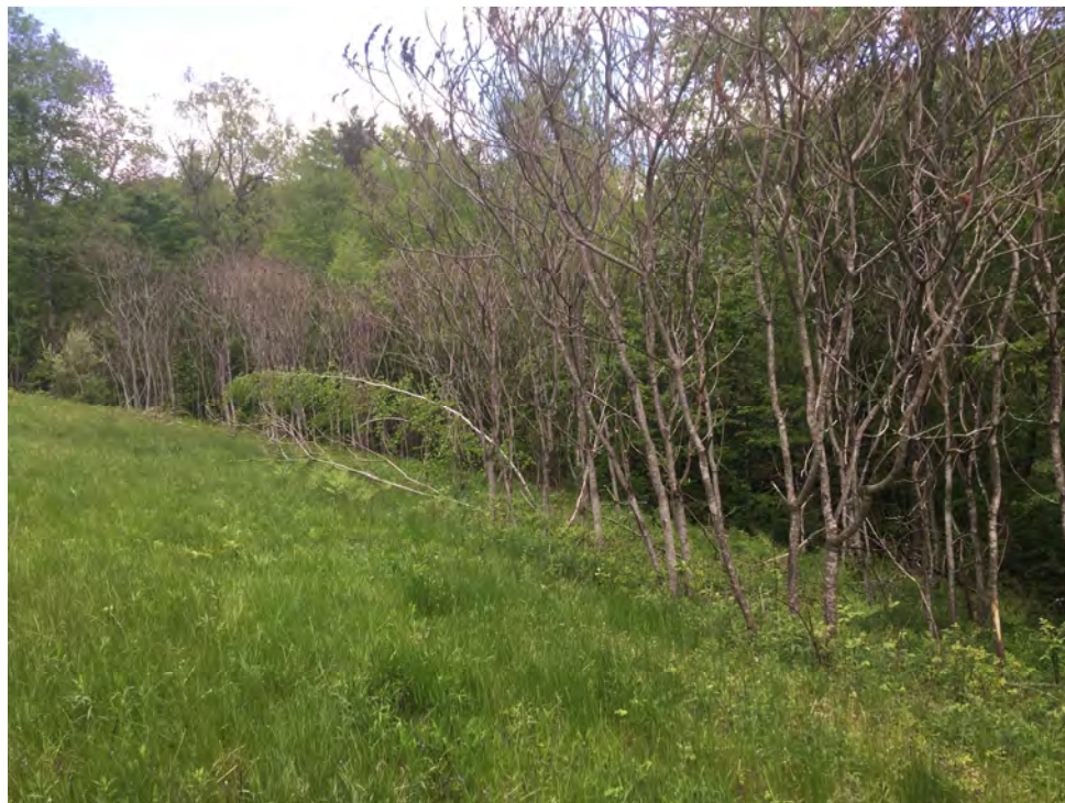
Photo 3 (looking north): Middle Closed Landfill area in fair condition. Sumac and small trees need to be removed from the landfill cap.
