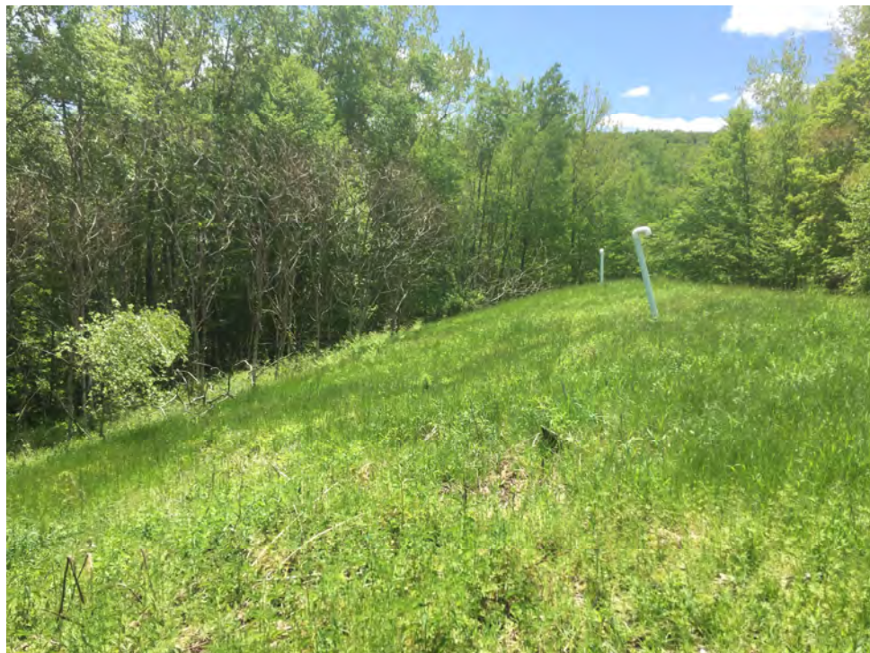
Photo 4 (looking south): Gas vents and top of closed landfill in fair to good condition.
