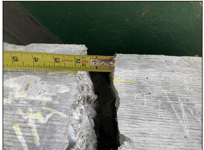
Wingwall #4 Settlement Crack
