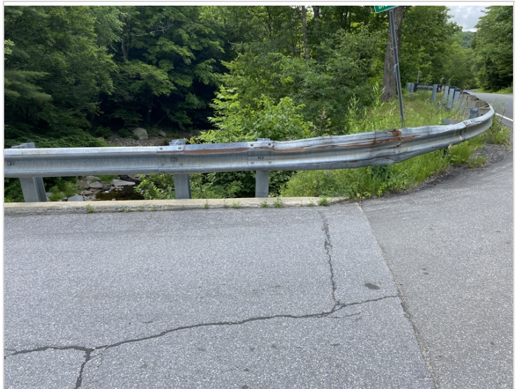
Downstream Transition Rail
