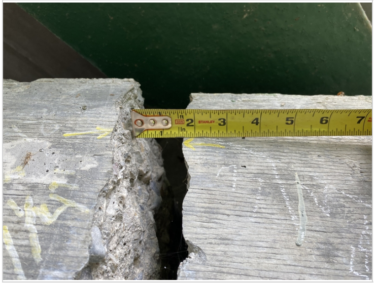
Wingwall #4 Settlement Crack
